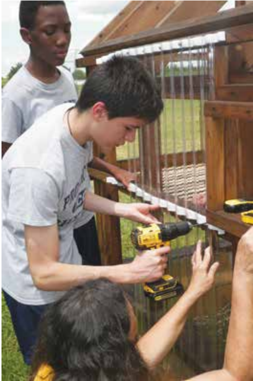
One of the ongoing projects has been the construction of the school's own greenhouse. Here, students complete part of the work.
